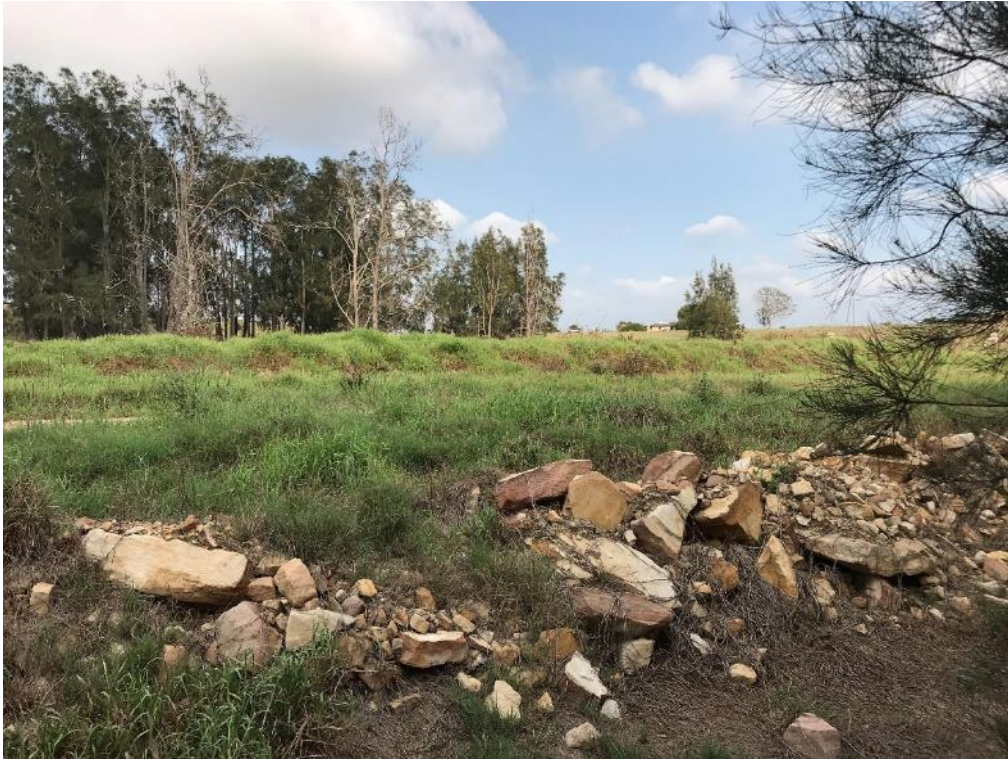
Plate 4.6 Fill used to create a level surface for the road. Bund beside dam behind. View north west.
