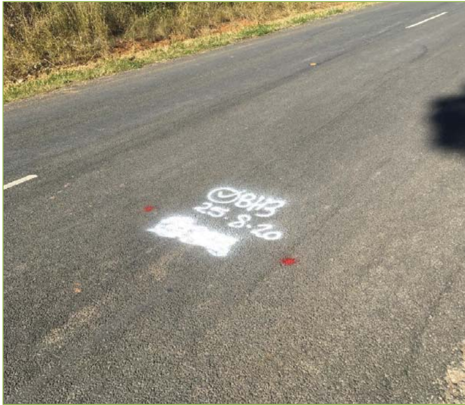
Figure 2.2.7 – BH3: Pavement Surface Condition
