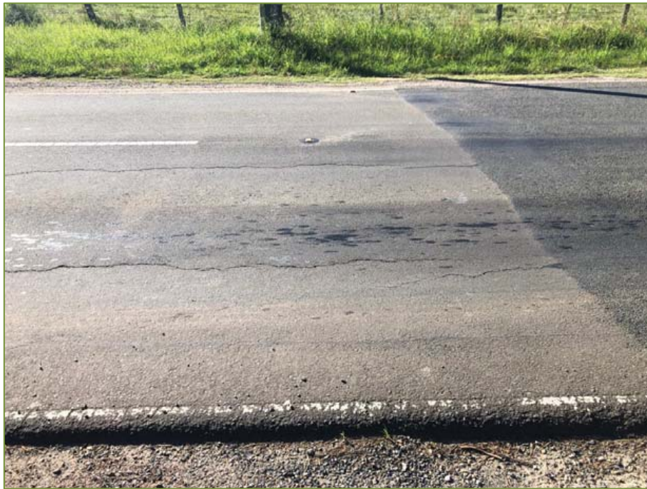
Figure 4.2.1 – Longitudinal Cracking CH35
