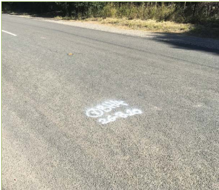
Figure 2.2.10 – BH4: Pavement Surface Condition
