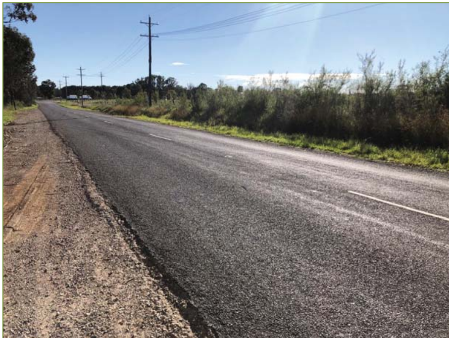
Figure 4.2.3 – Sprayed Seal Surface with edge drop off CH150.
