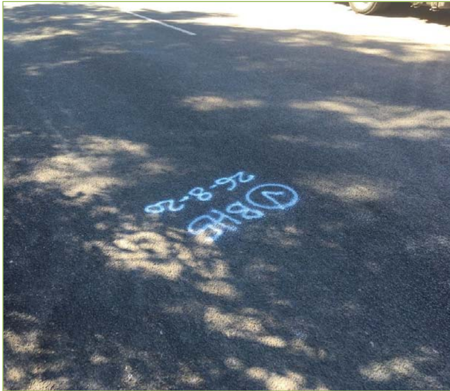
Figure 2.2.13 – BH5: Pavement Surface Condition
