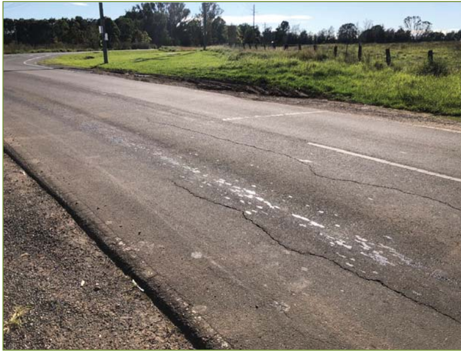
Figure 4.2.2 – Longitudinal Cracking CH30
