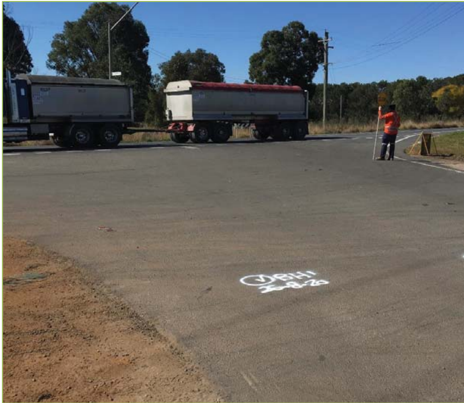
Figure 2.2.1 – BH1: Pavement Surface Condition
