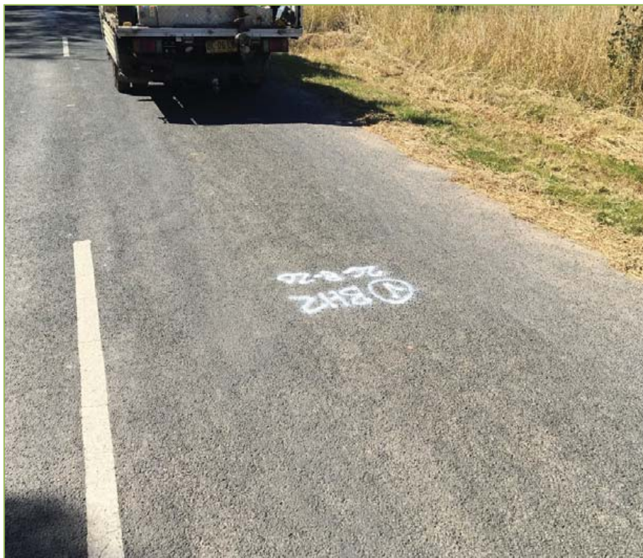
Figure 2.2.4 – BH2: Pavement Surface Condition
